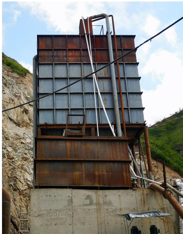
300m 3 絮凝沉淀罐
